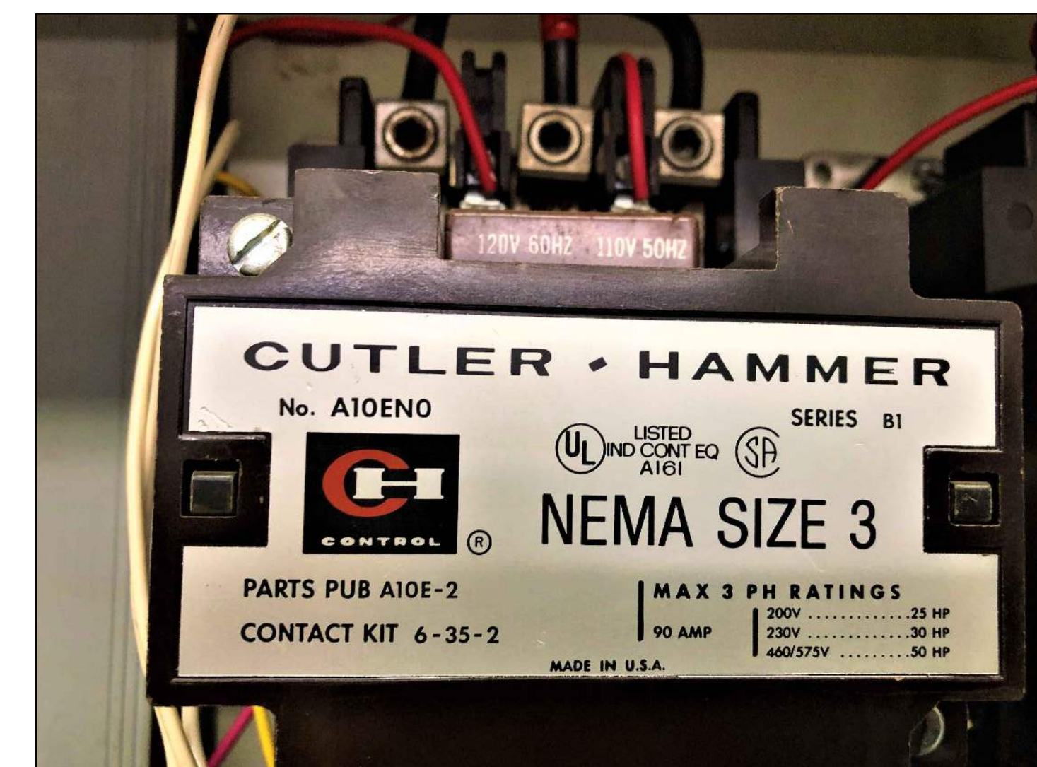
EXISTING MOTOR CONTROLLERS TO BE REPLACED BY VFDS
